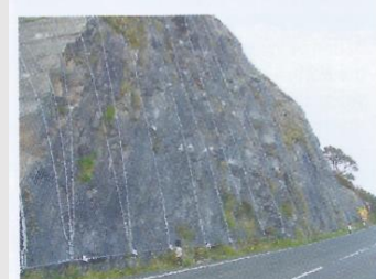
Figure 2 Rock bolts and wire netting
